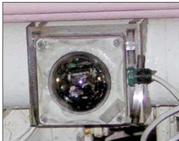
Figure 3. Photograph of an installed CCTV camera on F/T Seafisher encased in a cast aluminum armoured dome, showing stainless steel mount and band straps.
